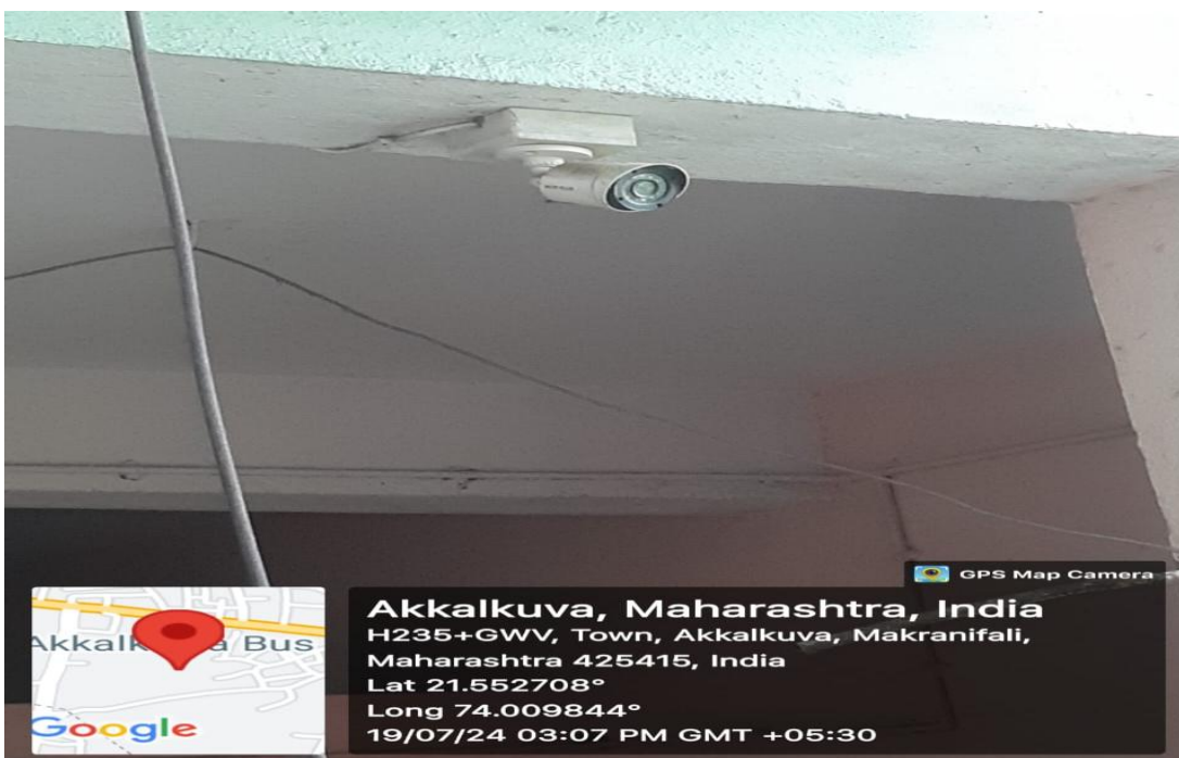
PHOTO OF CCTV
